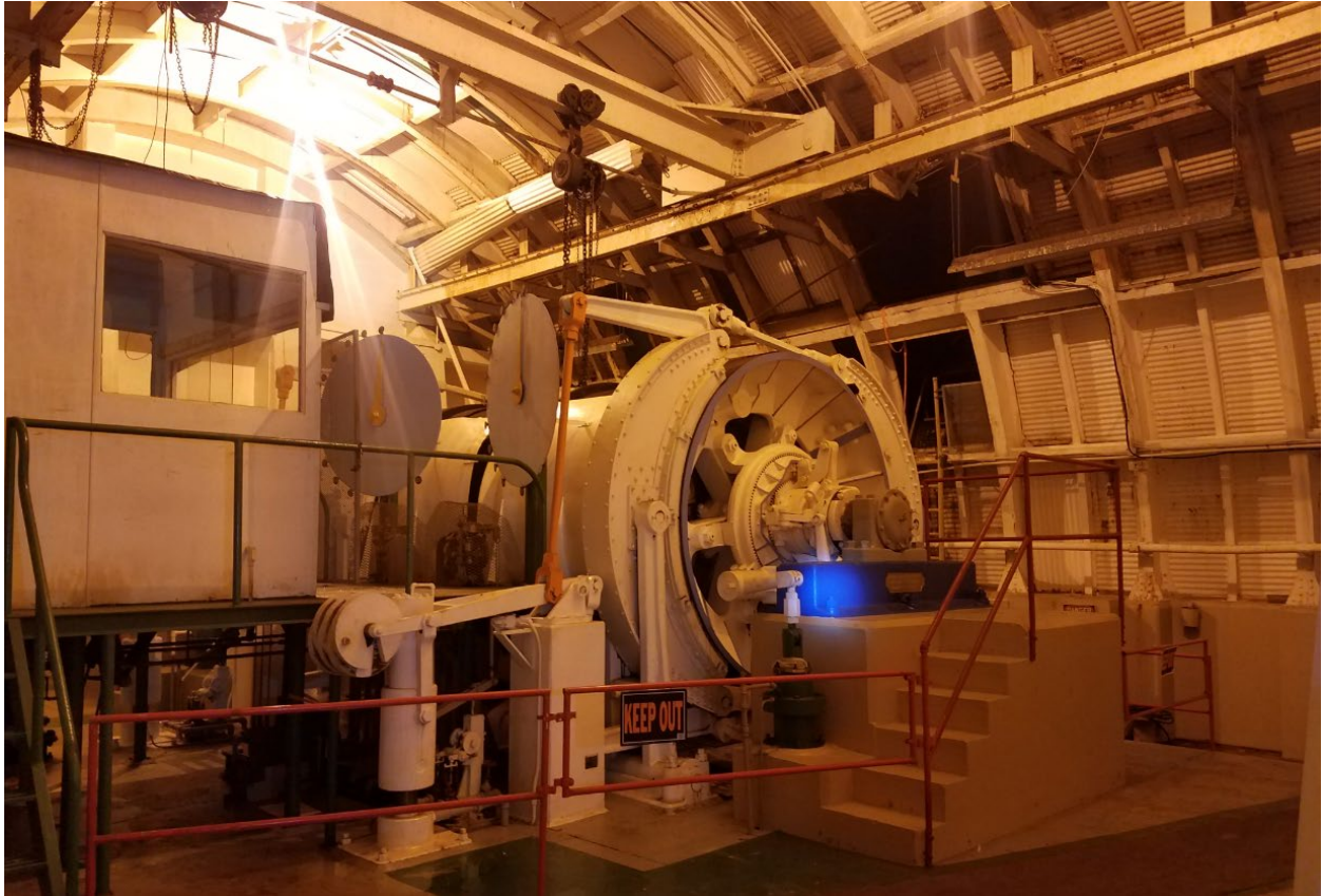
Figure 18-8 #2 Shaft Double Drum Hoist Room
