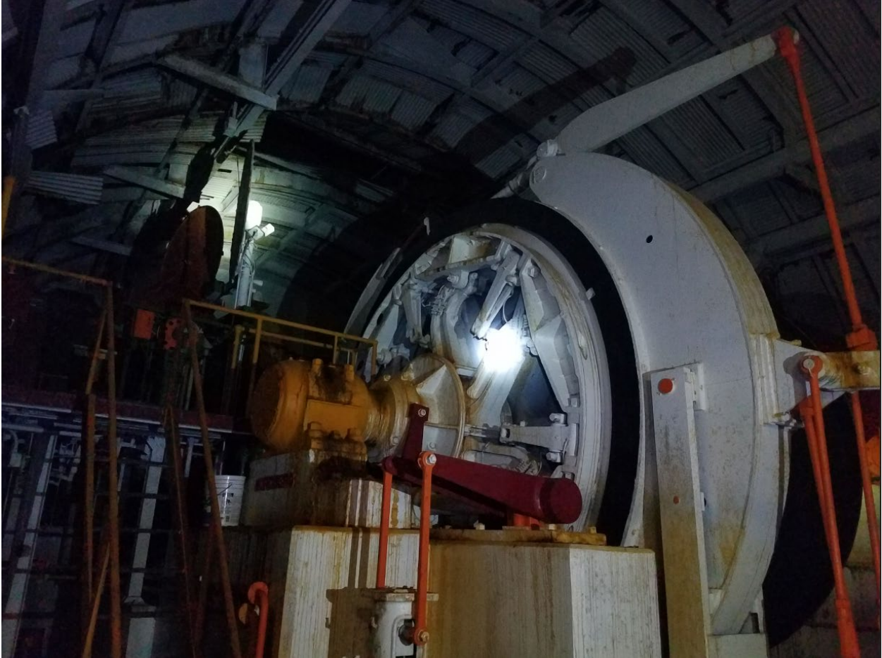
Figure 18-3 #1 Hoist and Hoist Room 9-Level
