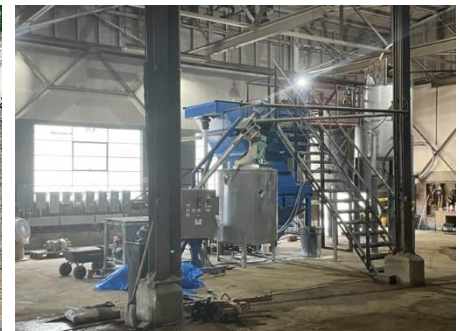
Photo 9: Pilot water treatment plant at Bunker Hill Mine
