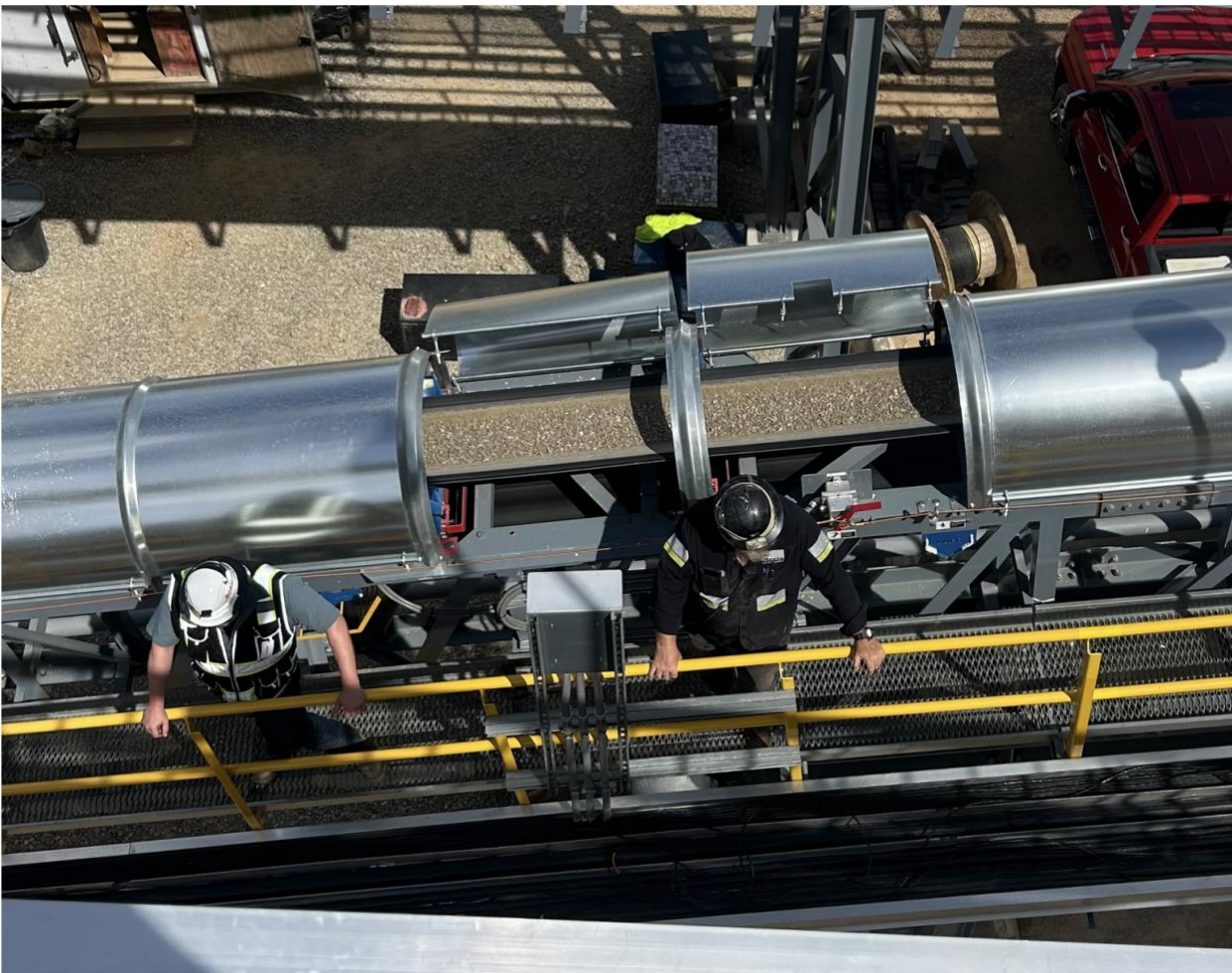
Figure 2: Crushed ore being transported to the Fine Ore Silo
