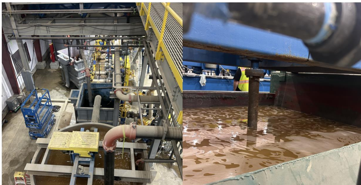
Figure 3: Water pumped through flotation and thickening circuits, ready for reagent and ore
