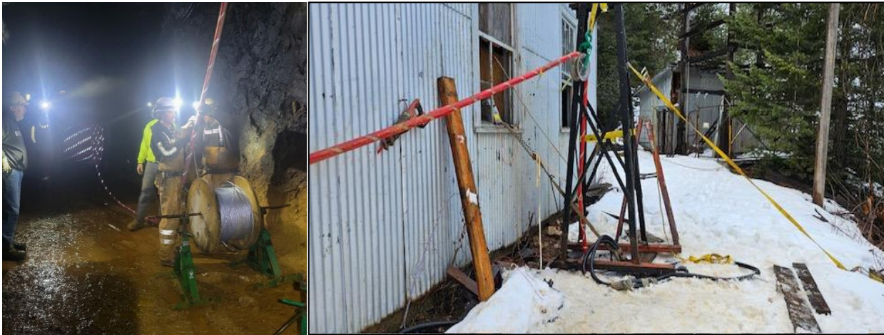
Power being 'dropped' from the Cherry Raise (R) underground to the 5 Level (L)
