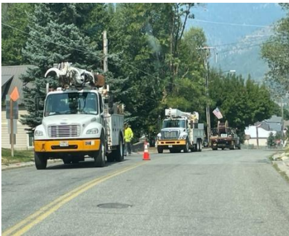
Figure 1: Avista Utilities working to install upgraded power from the nearby substation up Division Street in Wardner and to site.
