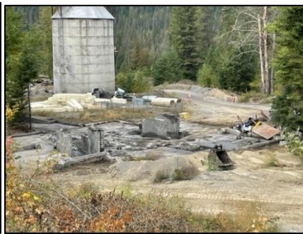
Photo 2: Crusher building reduce to its foundations
