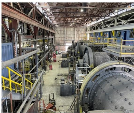
Figure 1: Ball Mills & Regrind Mill in main Mill Building (pre-dismantling) at Pend Oreille
