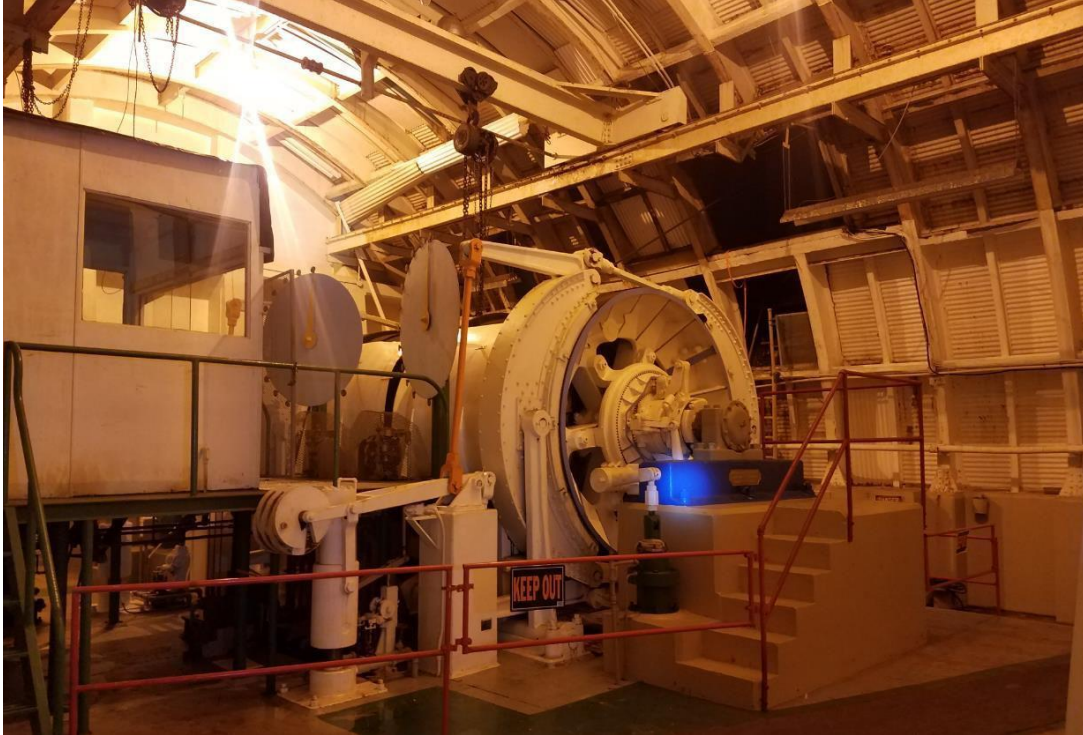
Figure 18-8 #2 Shaft Double Drum Hoist Room
