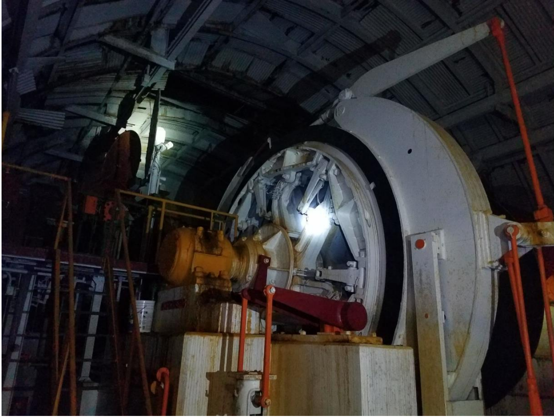
Figure 18-3 #1 Hoist and Hoist Room 9-Level
